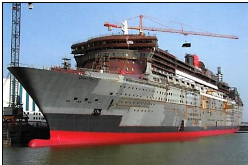
Saint Nazaire: Lowering the upper part of the funnel into position on April 4, 2003.
